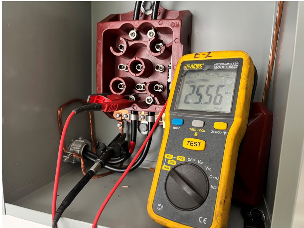
Figure 3. Insulation Resistance Test (Megger) of an airfield lighting circuit at the S1-Cut-Out
