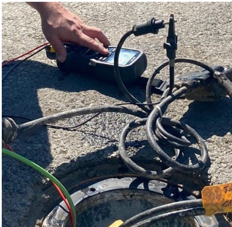
Figure 2. Meggering an airfield lighting circuit to find a fault in the field
