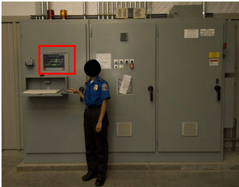
Figure E-1 BHS OPERATION UNIT
