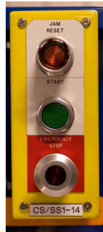
Figure E-23 CLEARING THE 'FAIL-SAFE' FAULT BY PRESSING THE START BUTTON
