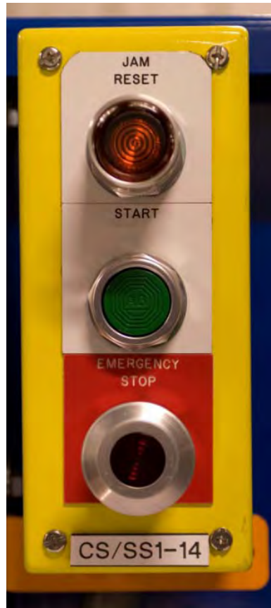
Figure E-25 RESTARTING THE BHS
