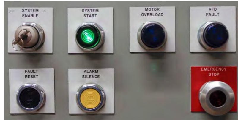
Figure E-2 THE BHS MAIN CONTROL PANEL
