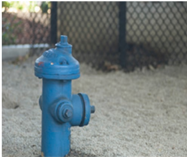
FIGURE 21 Fire hydrant in SFO SARA (SFO photo).
