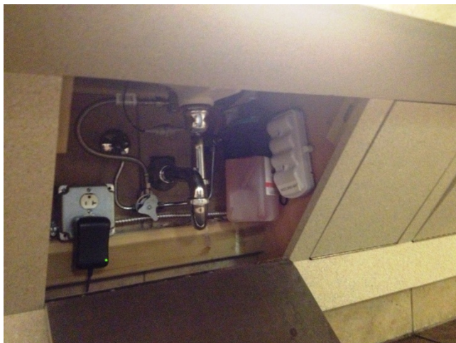
Access to Refill Soap, Traps, and Electrical Below Sink
